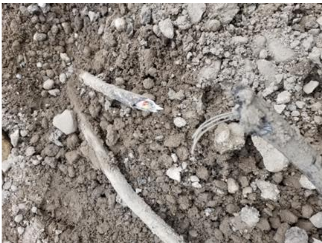
Perished Underground Electrical Cabling
